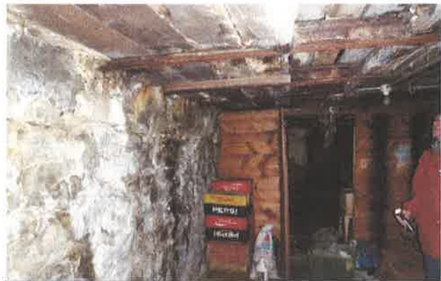
Photo #2: Callender St. Vault Wall and Lid
