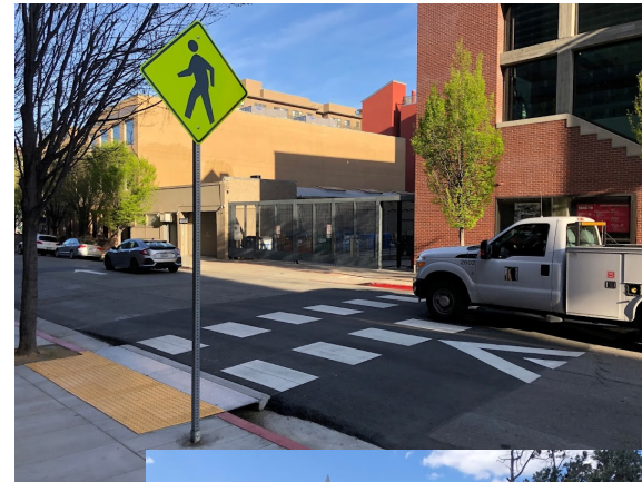
Mid-block raised crosswalk examples showing a bridging of the gutter (top) and in combination with a curb extension (middle).
