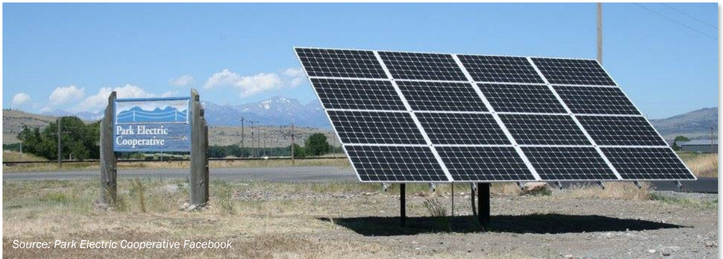
Figure 9.1: Park Electric Cooperative
