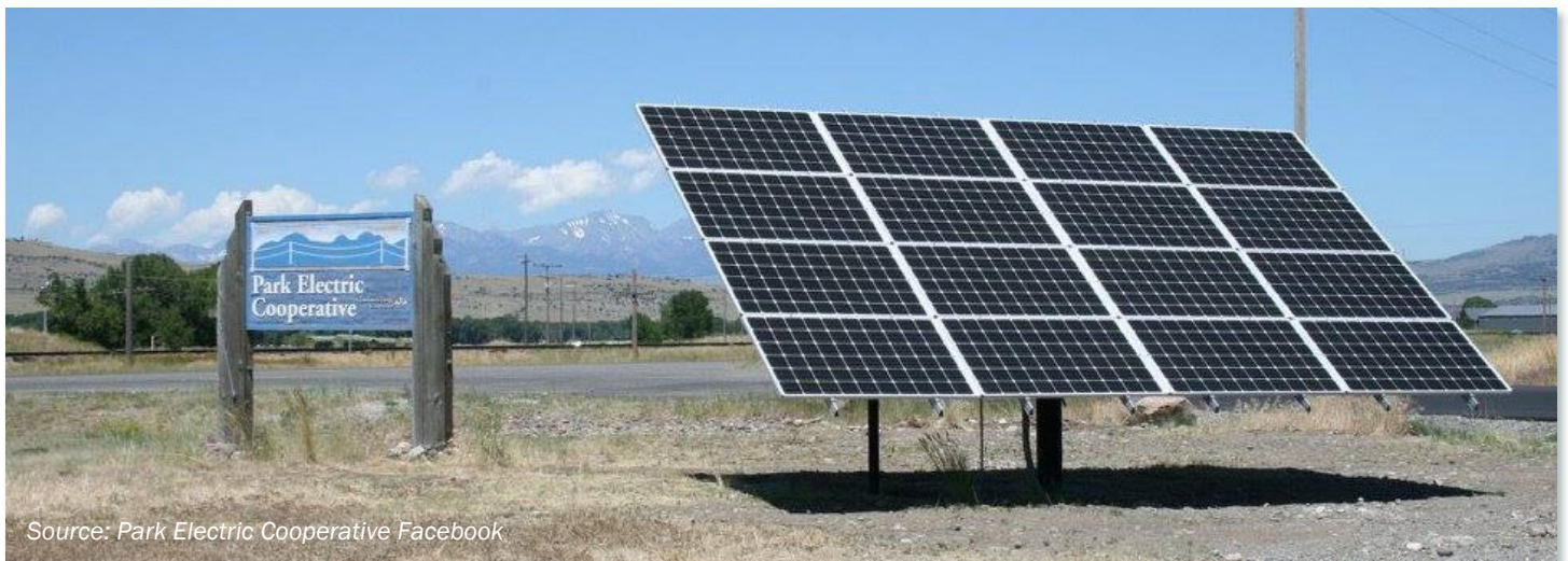
Figure 9.1: Park Electric Cooperative
